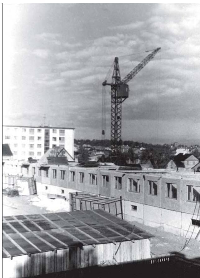
Photo 4. Newspapers of 1960s and 1970s reflected the building of blocks as a metaphor of building up communism. Tower crane and concrete blocks were signs of progress. New Tartu was built the same way. Year 1967. Photo by Urmas Karu.
