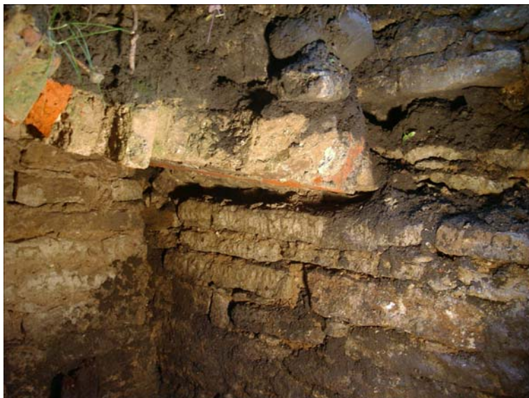
Figure 13. The cylinder vault of the burial chamber of the von Adlerbergs. The vault has been supported by the incised grooves in the long walls of the chamber and covered with soil.
